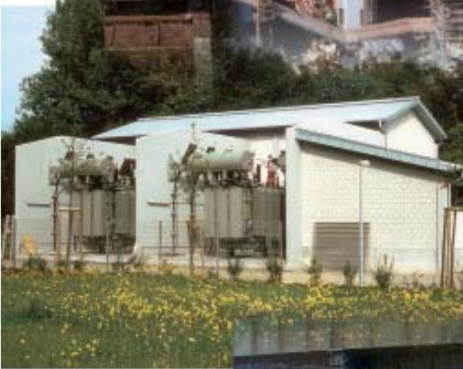
Application Public power supply system
